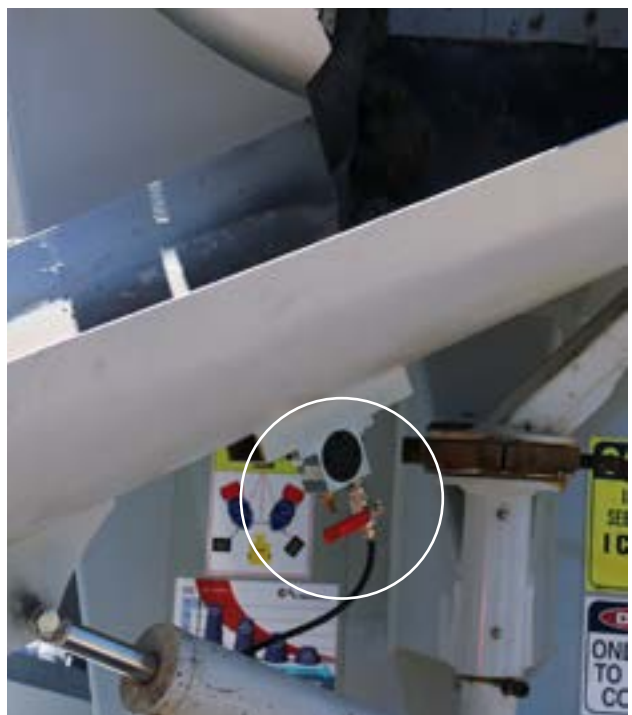
OT (rotary pneumatic vibrator) - Chute on concrete mixer
