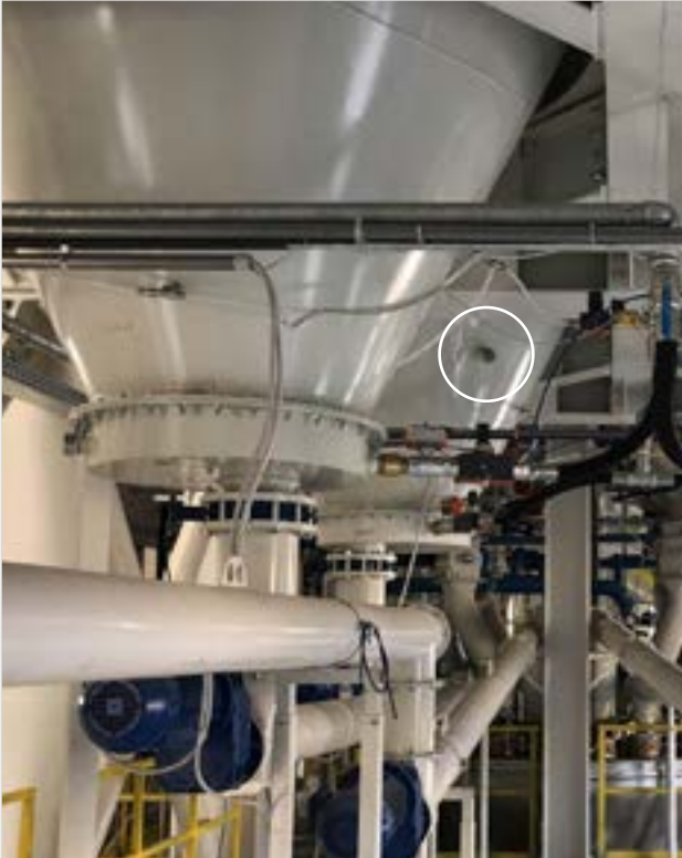
VBS (aeratoren) - Silos
