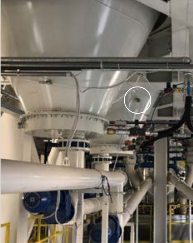
VBS (aireadores) - Silos
