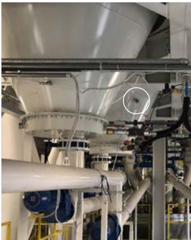
VBS (aeratori) - Silos
