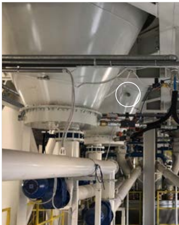
VBS (areator) - silosy
