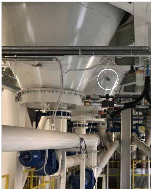
VBS (areator) - silosy
